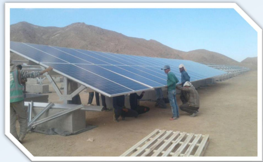
10 MW capacity grid-connected PV Power Plant (Fars Province, Iran)
