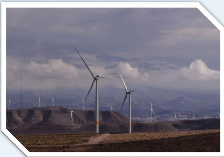
61.2 MW Wind farm (Qazvin Province, Iran)
