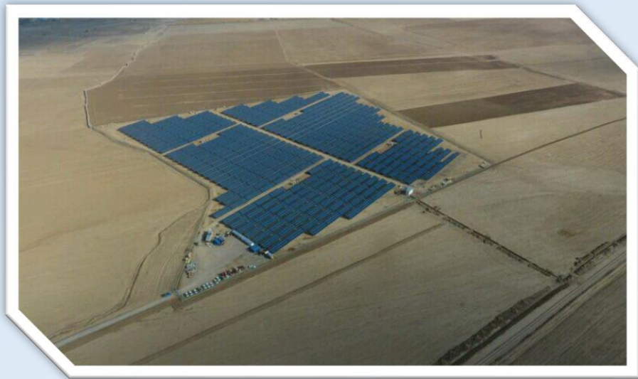
3×7, 8.9, 8.7 MW (total 38.5 MW) capacity grid-connected PV power plant (Hamadan Province, Iran)
